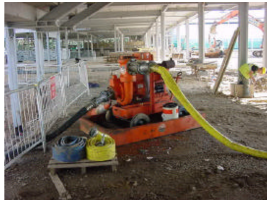
Suction pump to open tank
